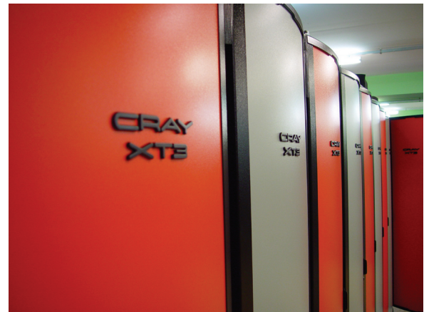
Figure 3: View of the Horizon system newly installed at CSCS.
